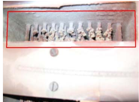
Typical deterioration above the burners
