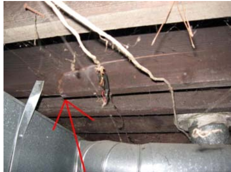
Large crack at floor joist
