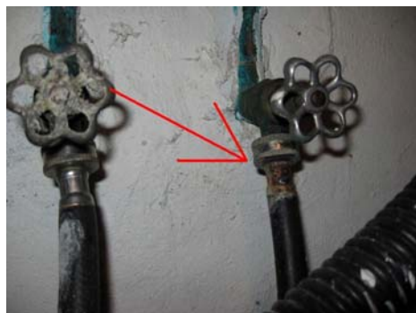
Leaking washer connection
