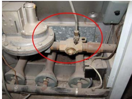
Area of gas leakage
