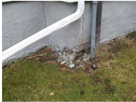
Deterioration at foundation
