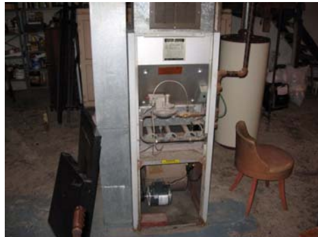
Forced air furnace
