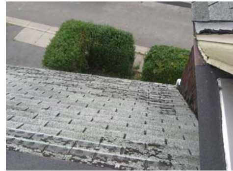
Weathered / damaged shingles
