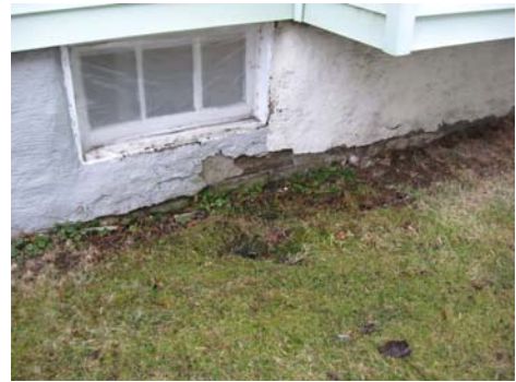
Deterioration at foundation
