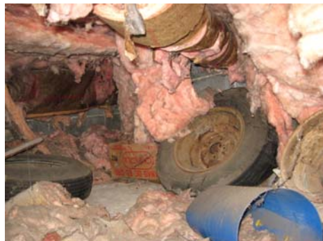
Falling insulation in crawl space
