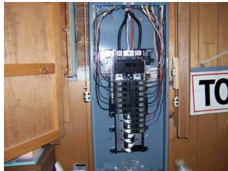
Main electrical panel
